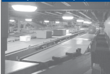
Photograph 5. The merge system
