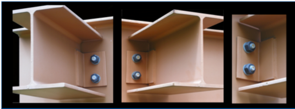
FIGURE 7 Close-up views of steel connection circled in Figure 4
